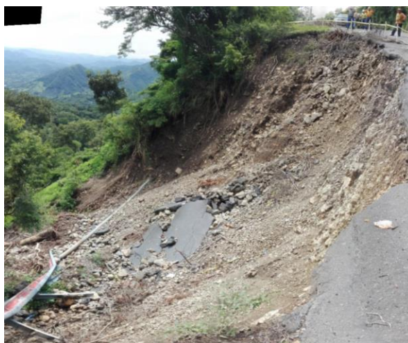
Figure 6.9 Road landslide to the turns, Chalatenango 2016. (MOP El Salvador)
